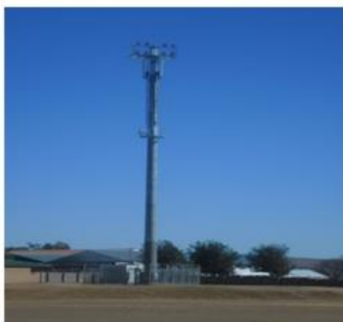
HIGH MASTS LIGHTS WARD 4
